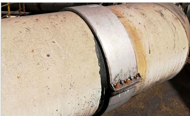
05 In service · running on a chemical plant line
